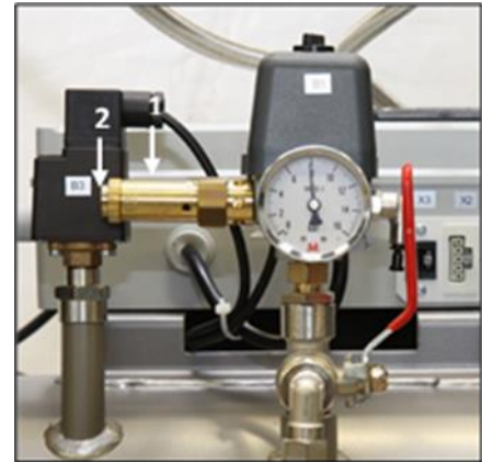
Fig. 17: Check of safety valve
